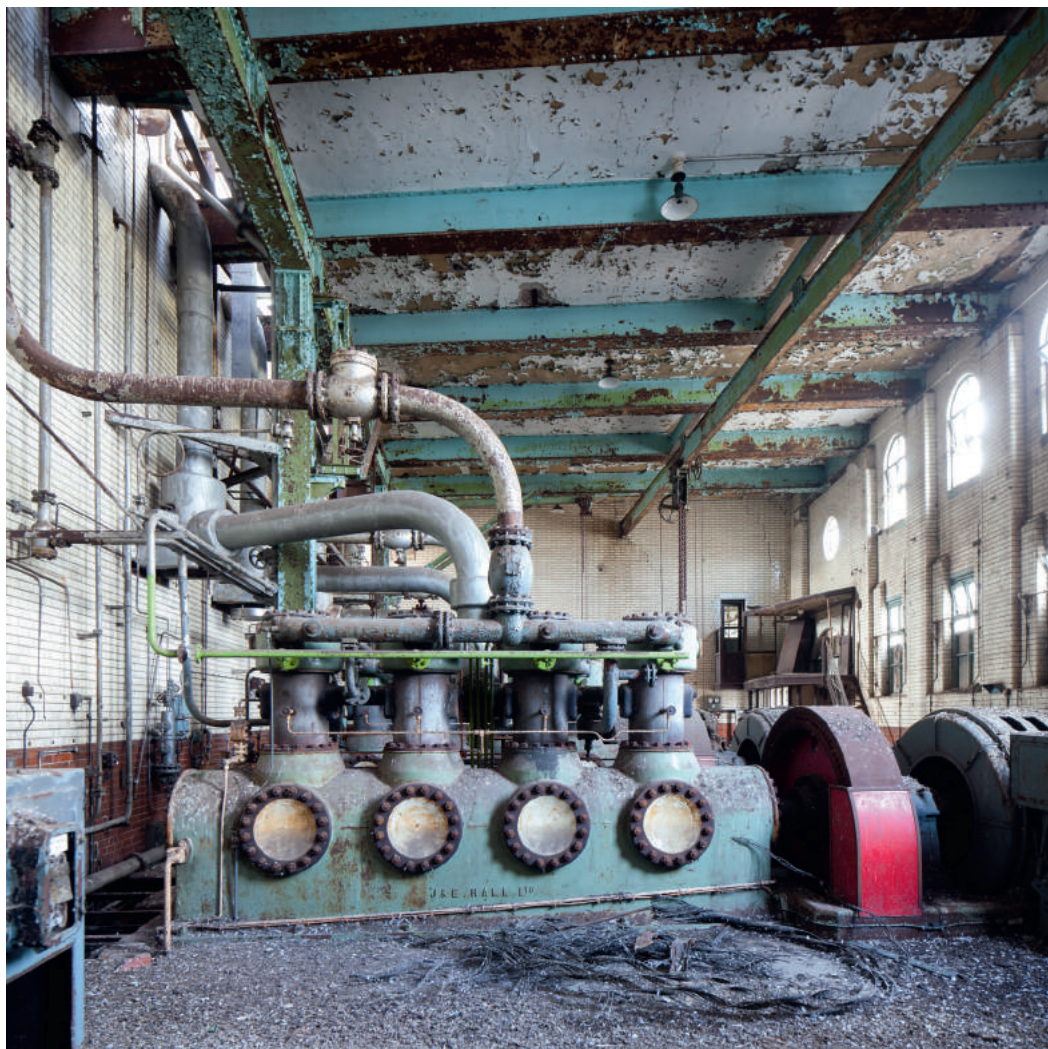
Machinery inside the Ice Factory (Image: Andy Marshall/World Monuments Fund)
