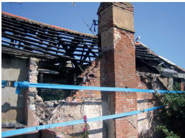
The roof of Castle House before and after the works had started
