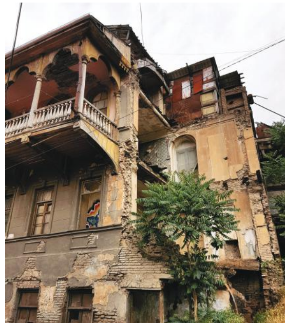
A collapsed building in the Avlabari district
