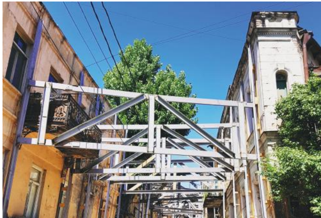
The area around Gudiashvili Square is currently held up by steel supports
